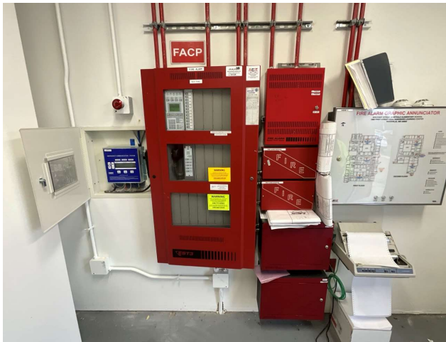
21 - FIRE ALARM PANEL
