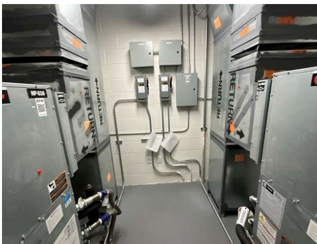
23 - INTERIOR HEAT PUMPS
